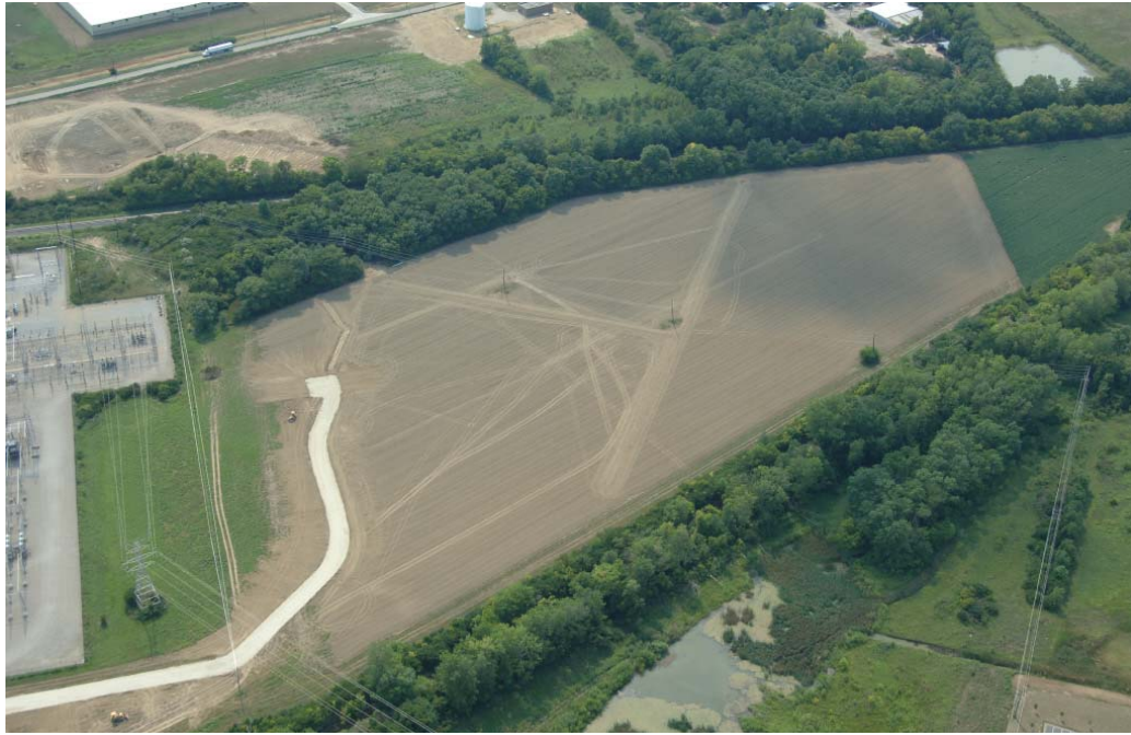
Construction at the facility began on August 1, 2007. This photo is the first aerial photo after the access road was installed and the soil was turned at the facility.
