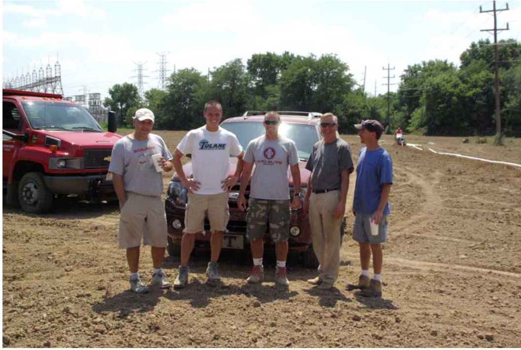
Girls Director of Coaching Doug Bracken is joined by Kurt Hutter, Nick Flohre, Bill Reagor, Dan Seig, Tim Smith (not pictured) and Scott Leist (not pictured) spend a day at the facility installing over 1400 ft. of irrigation piping. The pipe will help provide water to the fields.
